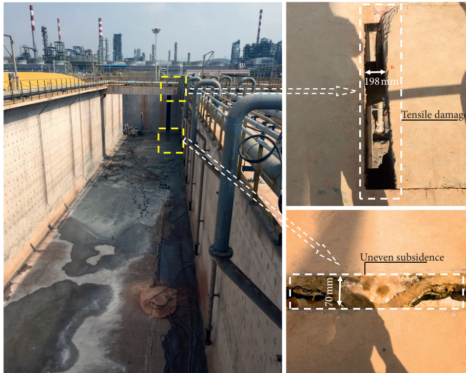
FIGURE 3: Tensile damage and uneven subsidence of the biochemical pond.
